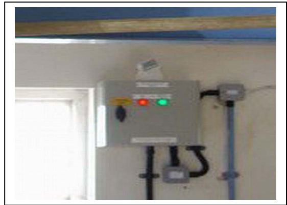
Internal electric connection with PIR security system to prevent mis-use of the system
