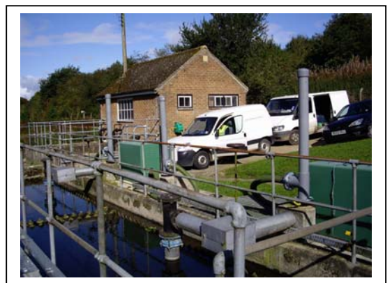
All installed and working in a 24 hour period supplying approx. 15,000 litres per year at this site.
