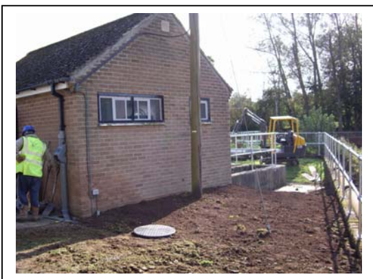
Transparent site now with a water supply for washing down equipment/pumps & servicing internal toilet
