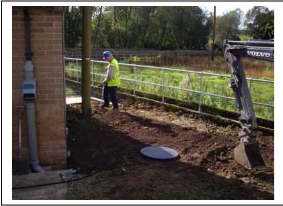
The flat tank is covered with top soil and has A lockable child proof cover
